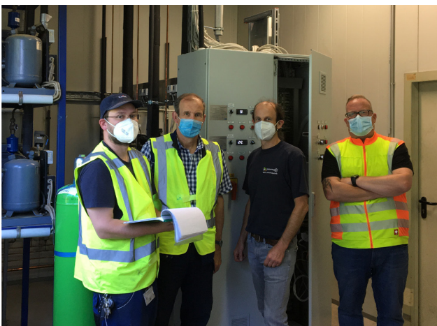
Handover of the completed refrigeration system in the plant room (refrigeration system in the background), from the left, Christopher Popp, Armin Klein, Ralph Rinck, Rene Lämmermann
