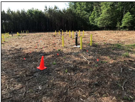
Photo 5: Layout of injection locations. MW-34 pictured in foreground.
