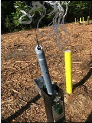
Photo 19: PlumeStop in bailed sample from one of the permanent monitoring wells in the area.
