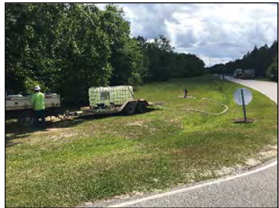
Photo 4: Hydrant water source located along the truck delivery route for Fayetteville Works.
